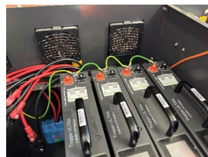
Daisy chain the earth cables (4 battery example)
