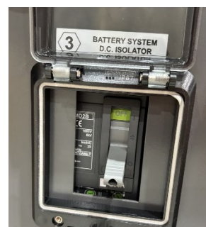
Battery System D.C. Isolator
